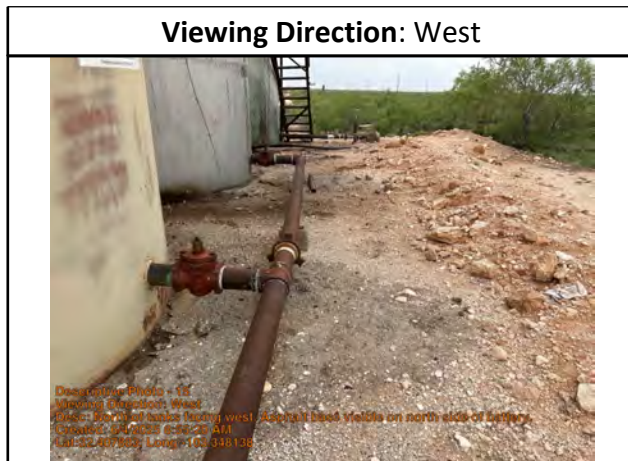
North of tanks facing west. Asphalt base visible on north side of battery.
