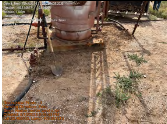
Heater treater west side
