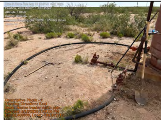
Heater treater north side
