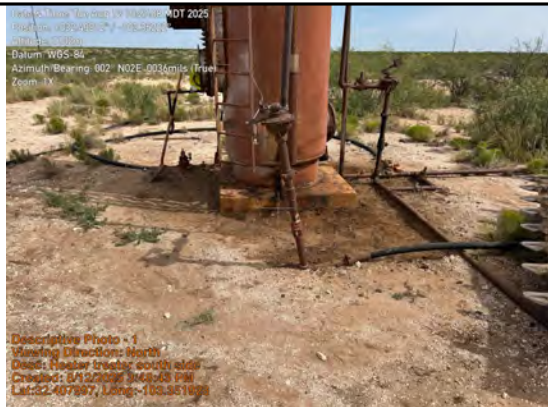
Heater treater south side
