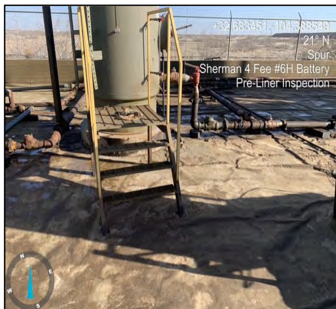
Photograph taken during initial assessment facing north.
