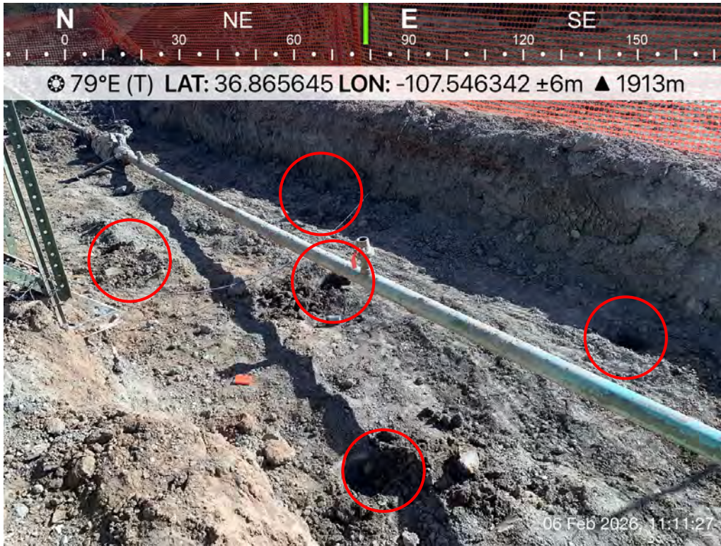
Photo 15: SS14 collected as a 5pct sample from the base of the POR excavation.
