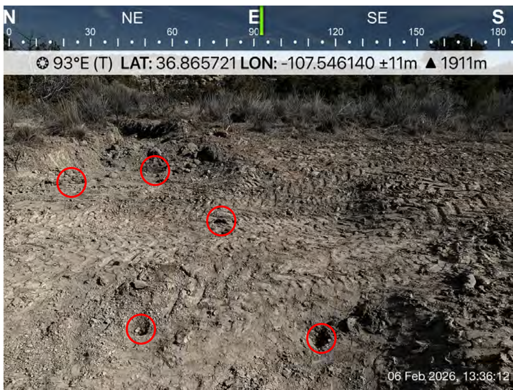
Photo 25: SS24 collected as a 5pct sample from the base of the release area excavation.
