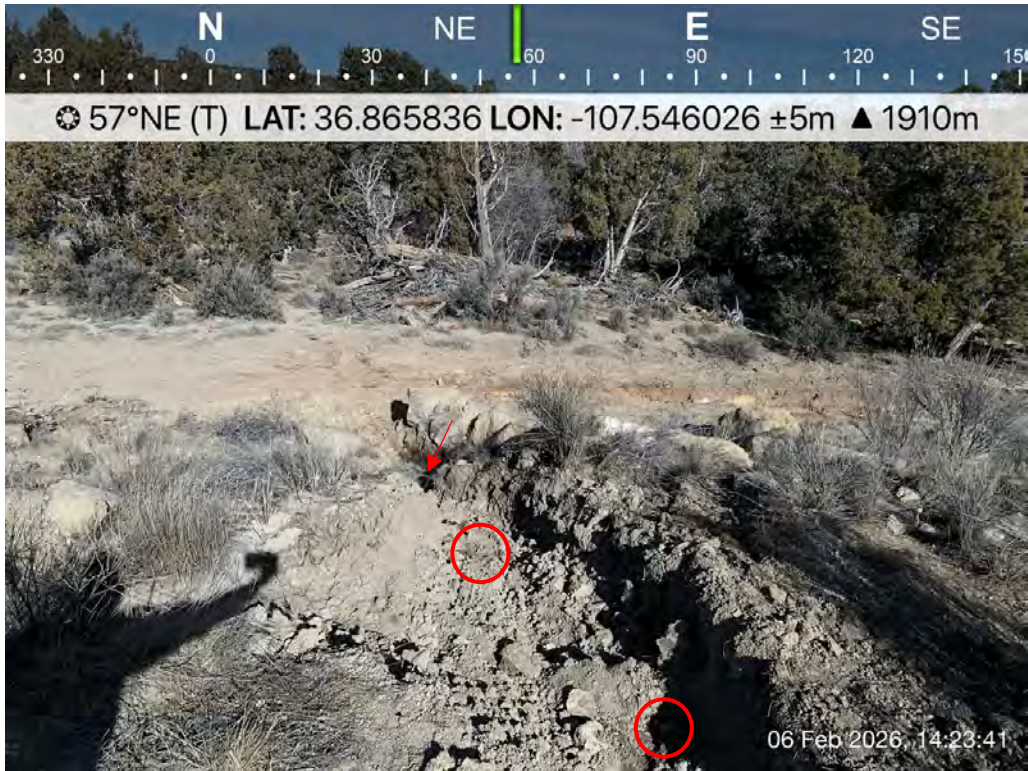
Photo 31: SS30 collected as a 5pct sample from the north fork of the release area excavation, some points not visible in the photo are denoted by the arrow.
