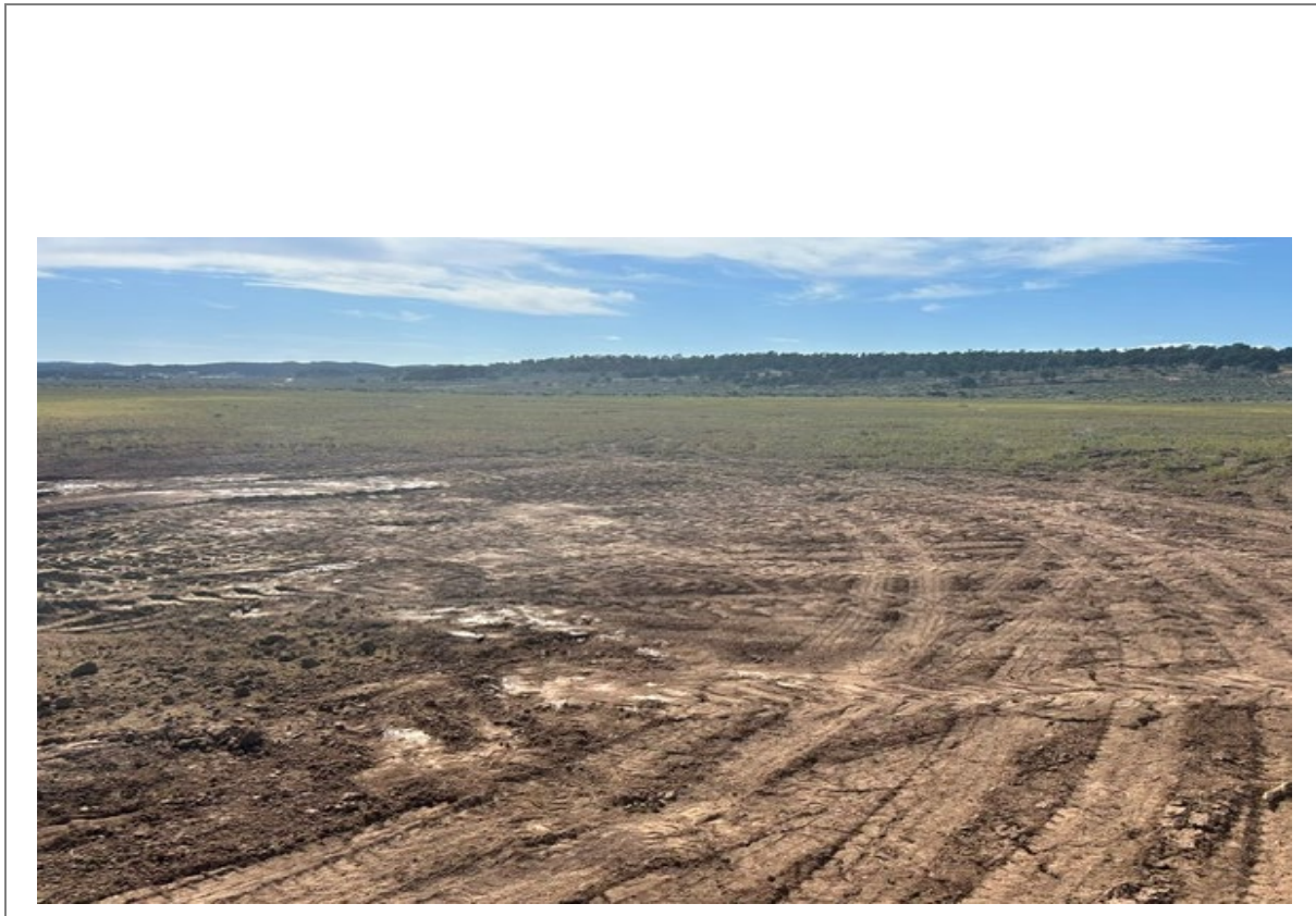
Photograph 8 — Post-excavation backfill and site restoration at the SB4 excavation footprint, McCroden Line release area. The excavation was backfilled with clean native borrow material, lightly compacted, and graded to match surrounding contours; the restored surface was prepared for revegetation consistent with the surrounding undisturbed upland-mesa rangeland.
