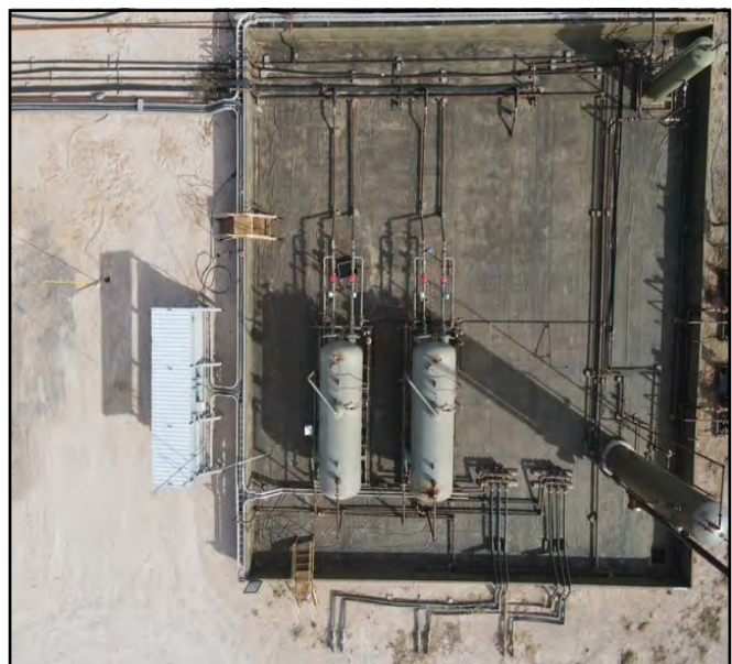
Aerial photo of initial assessment.
