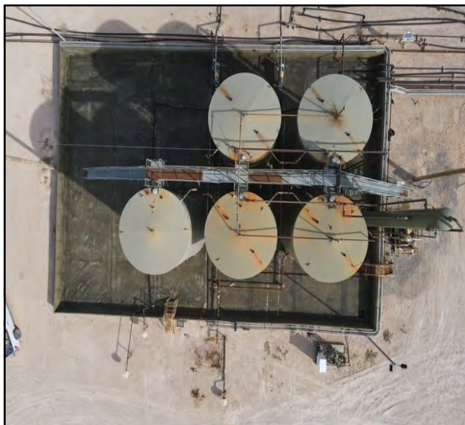
Aerial photo of initial assessment.
