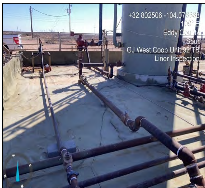
Photograph taken during initial spill release facing east.
