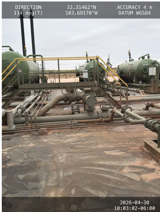
Photo 7 View of containment towards east-southeast.
