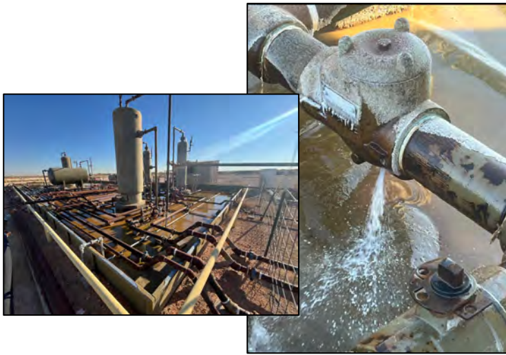
Photograph: 1 Date: 09/27/2025 Description: Initial release observed for Incident Number nAPP2527230287 POR located at approximately 32.09331°, -103.89309°
