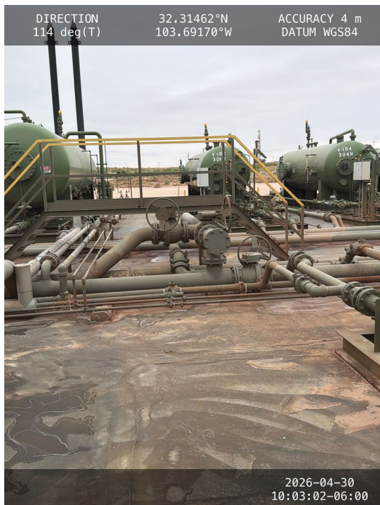
Photo 7 View of containment towards east-southeast.
