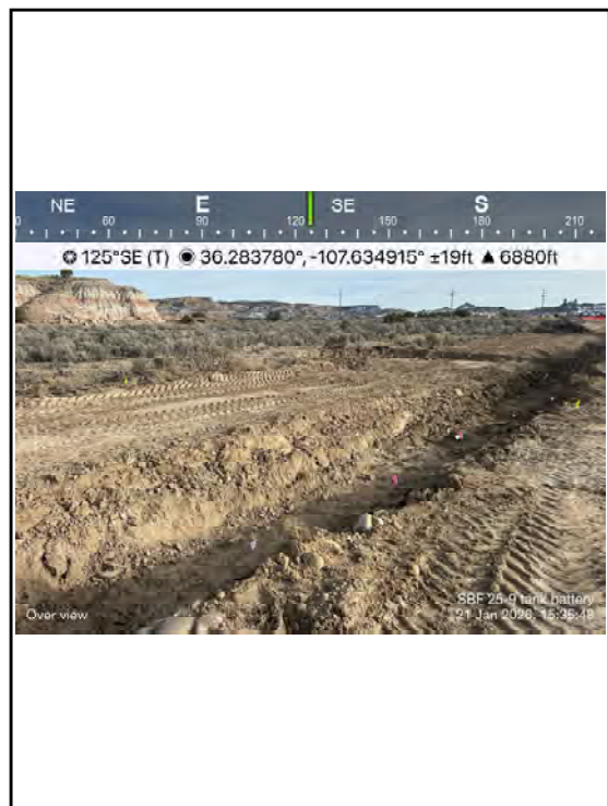
Photo 20 Excavation at north end of the release across the roadway and within the ditch following the access road.
