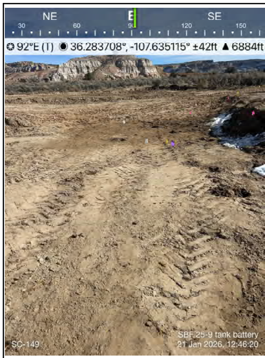
Photo 23 Excavation of the release area where it crosses the pipeline right of way on the north end of the release.
