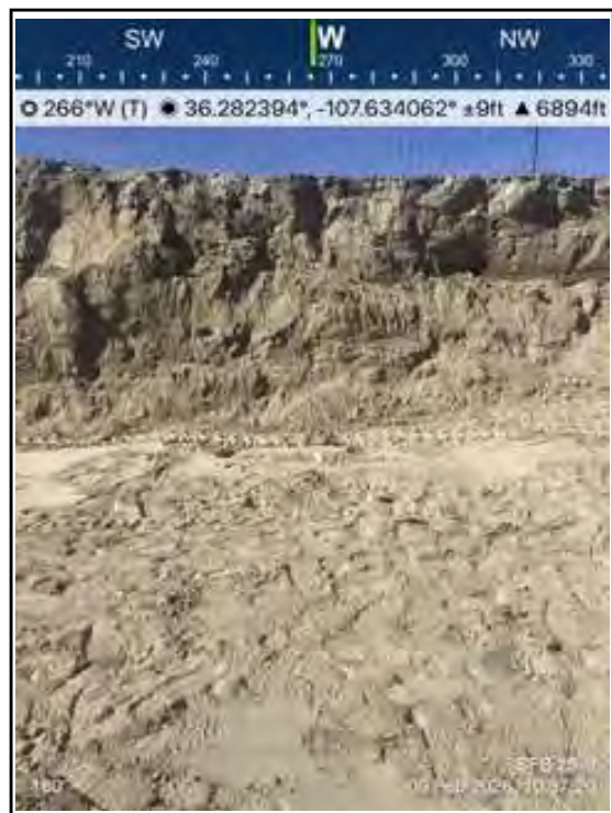
Photo 4 West wall continued on the main excavation below the former tank battery.
