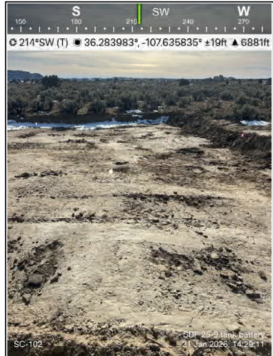
Photo 26 Excavation of the release area in the field at the end of the release pathway.
