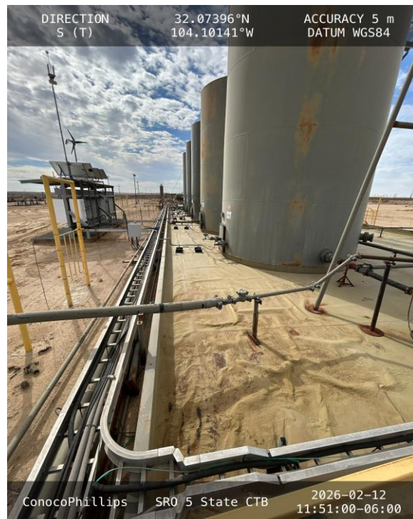
Photo 4 View of east side secondary containment towards south.
