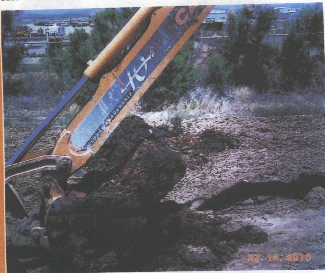
Below-Photo of Cell-2N-VZ-2 shows oily stained dirt about one foot under surface.
