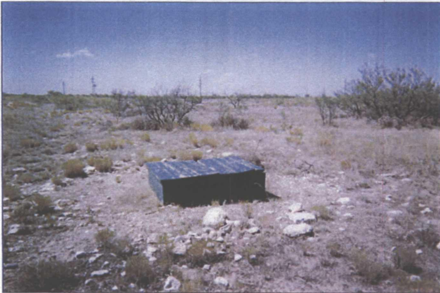
undisturbed junction box
