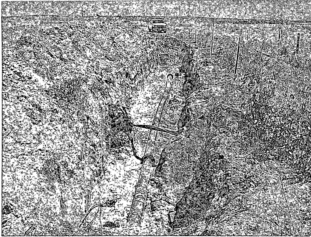
View east – mainline source (8/13/09)
