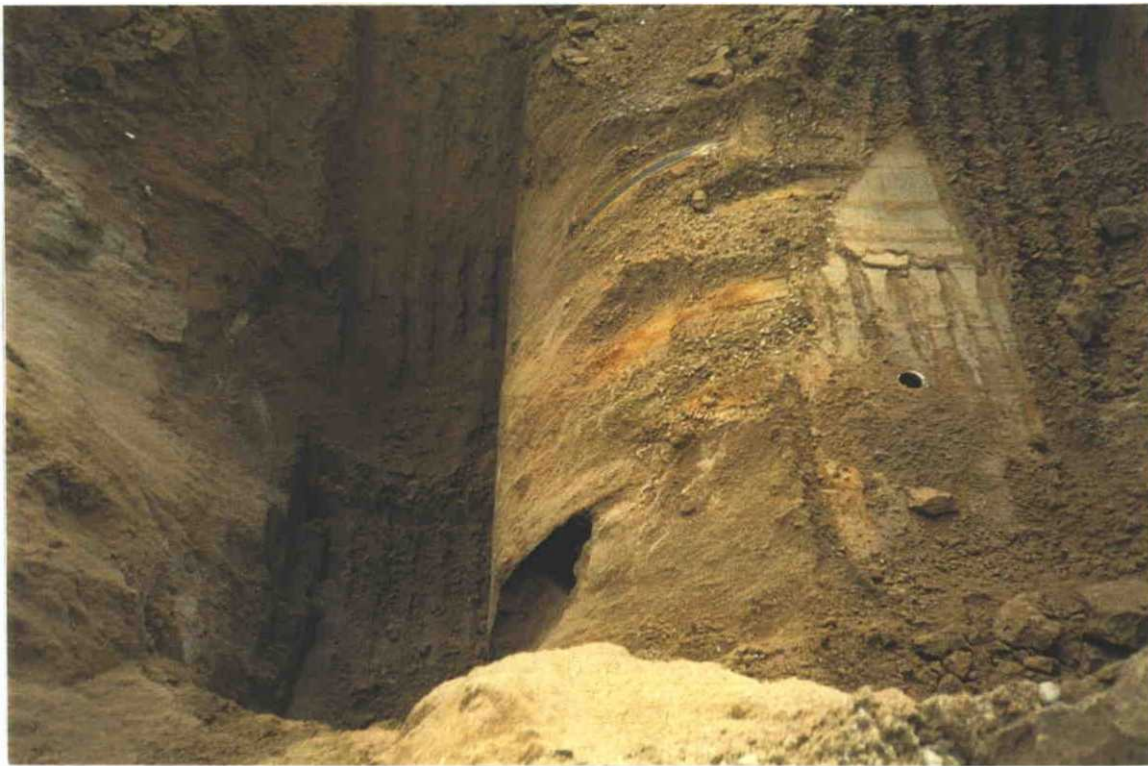
Photograph #9 Digging Beside the FWT; North End of Tank Showing (Collapsed inward)
