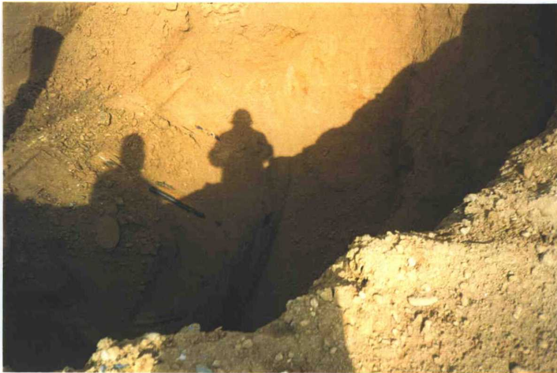
Photograph #8 Hole in the FWT
