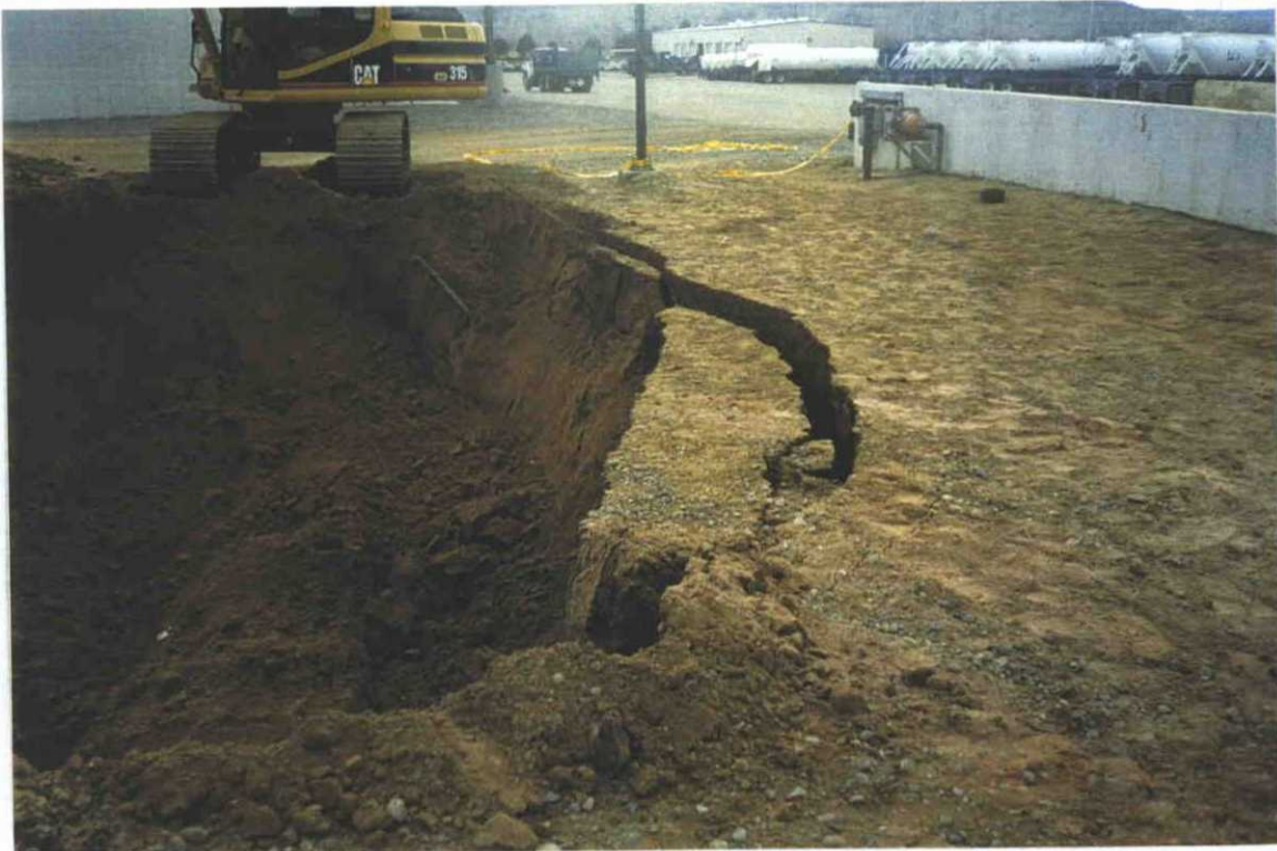
Photograph #7 West Wall of FWT Excavation Showing Excavation Instability
