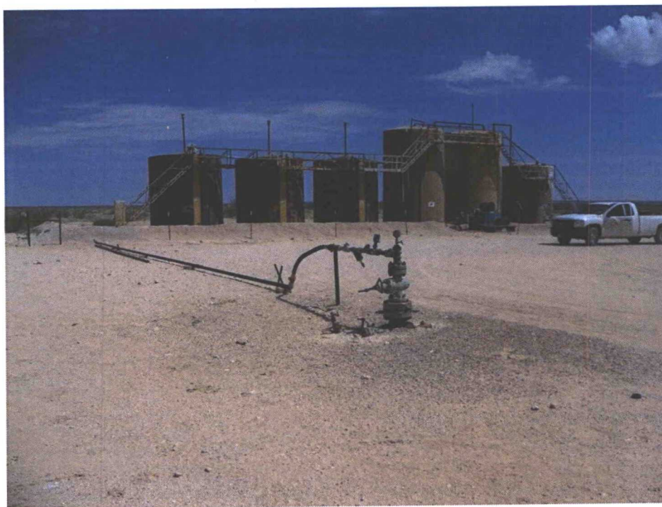
Photo 2: View of SWD Well and Tank Battery
