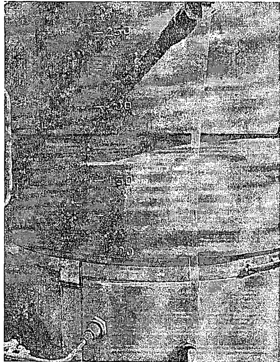
WAMs Unit close-up w/ manometer
