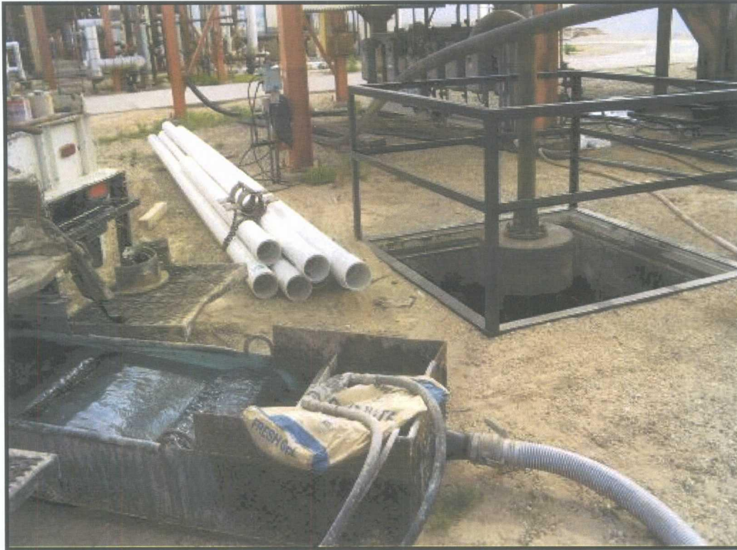
Cuttings separator box with oil, next to leak detection sump, April 2009
