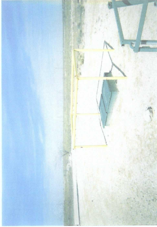
undisturbed junction box (1)
