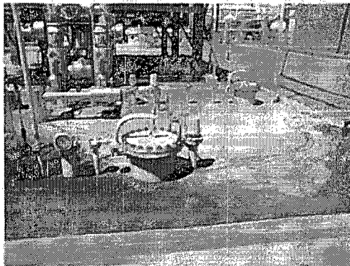
Pic #3 Amine Waste Sump area- Sumps are single wall.
