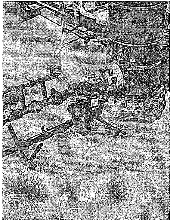
Rusty fittings near wellhead pinhole leak(s)?
