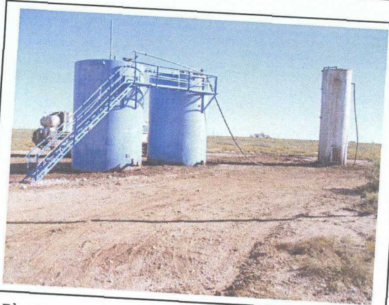
Photo of Tank Battery location looking northeast.
