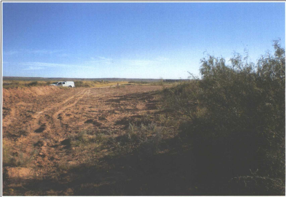
Photograph 6 Regraded area with the southern berm of Cell 6 to the left in the photograph and the southern and western berms of Cell 5 in the background behind the truck (view to the northeast).
