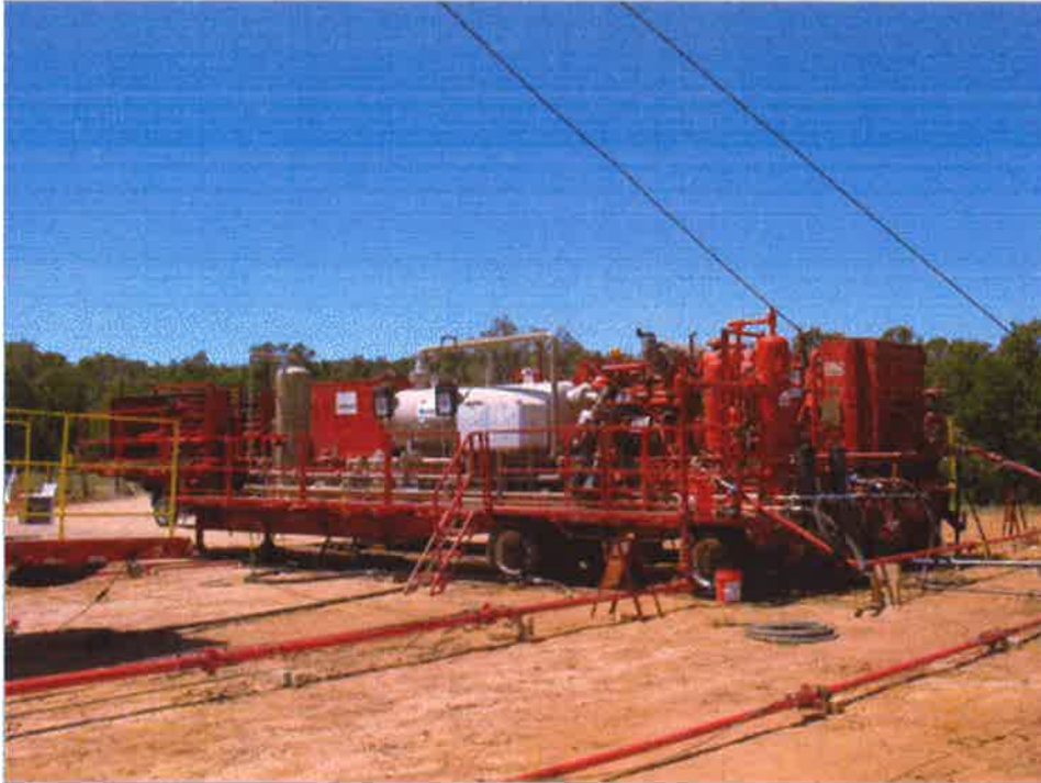
Figure 1. Truck-mounted green completions equipment. (Source: Weatherford. Natural Gas Star, 2010)
