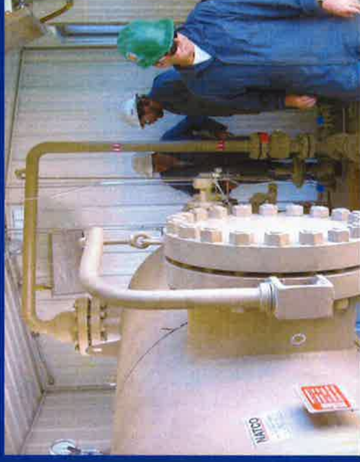
Portable Three Phase Separator, Source: BP
