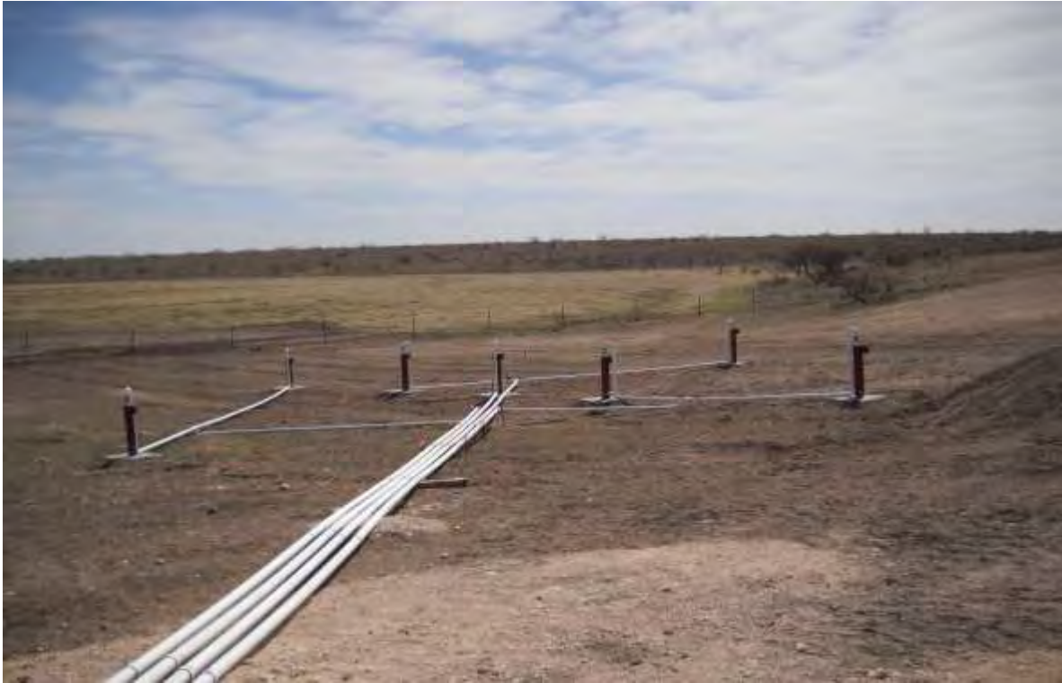
EK Queen Pearce 6-Inch – SVE Wells & System Piping (Looking Southwest)
