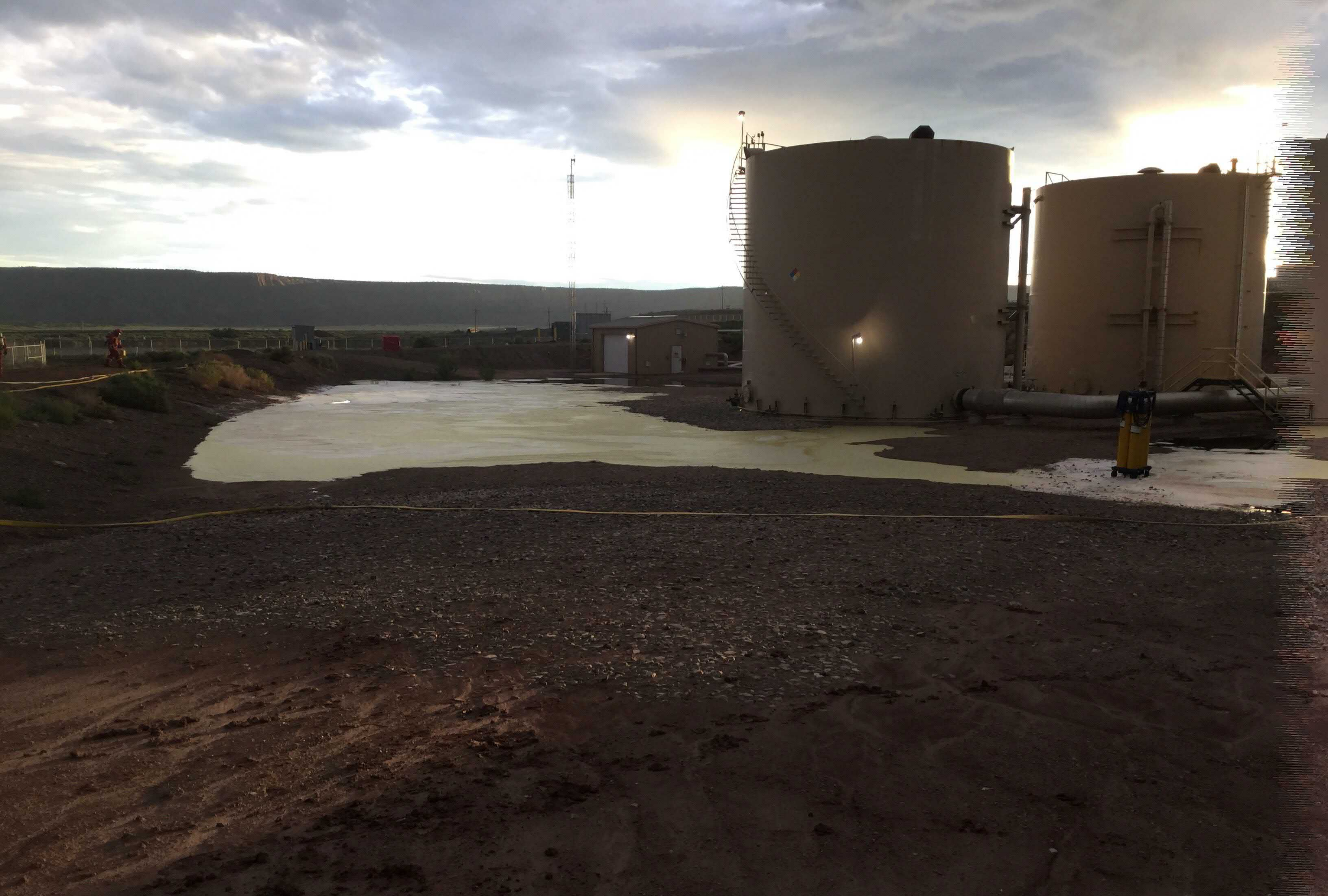
T-35 Tank Dike with Foam - Looking North
