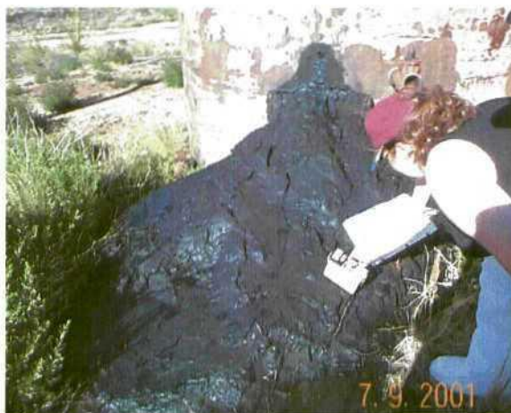
Photo 17. Tank #1 (north tank) with hydrocarbon material that has leaked out of a hole.
