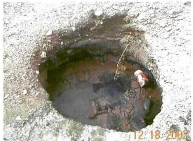
Photo 7: A sinkhole developing in the top of the pit that was located on Deck property north of the General Petroleum facility. General Petroleum operated this pit.
