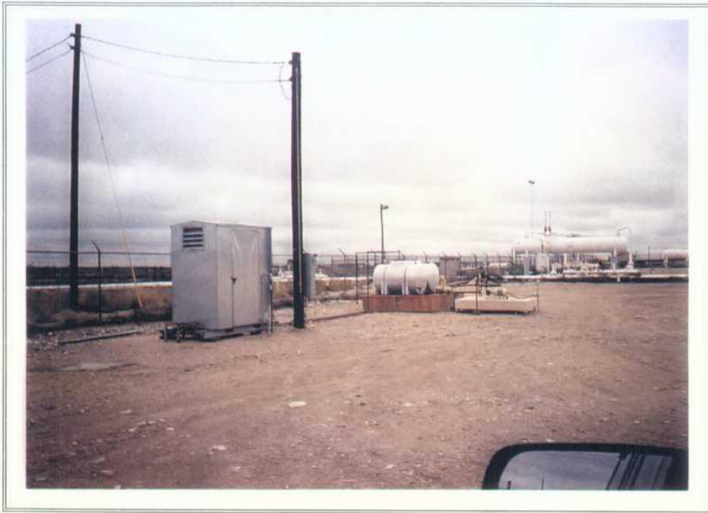
1. East Side Ferret System - storage tanks, transfer pump & compressor building.
