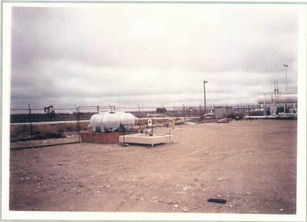
2. East Side Ferret System - storage tanks & transfer pump.
