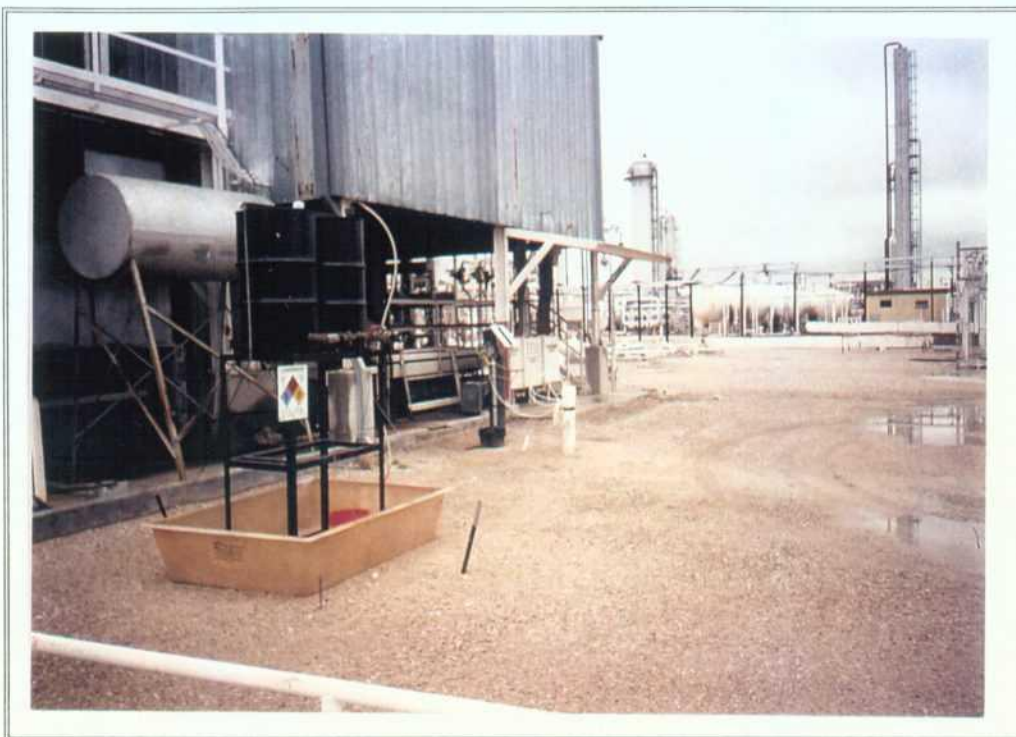
5. West Side Hydrocarbon Plume RW-2 – typical product storage tanks and controls.
