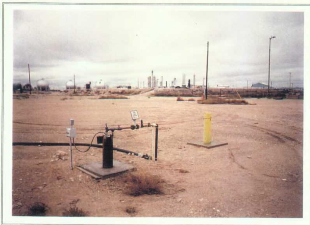
4. CRW-2 (MWD-9) - well with meter.
