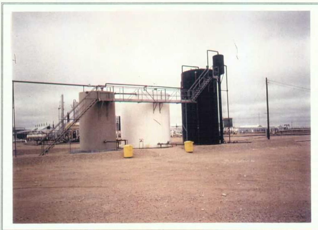
6. Eunice South Plant – separation and water storage facility.
