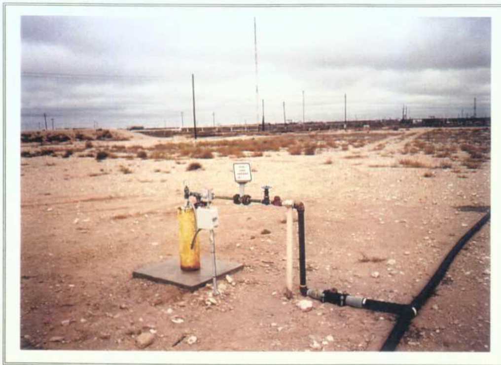
3. CRW-1 (MWD-3) - well with meter.
