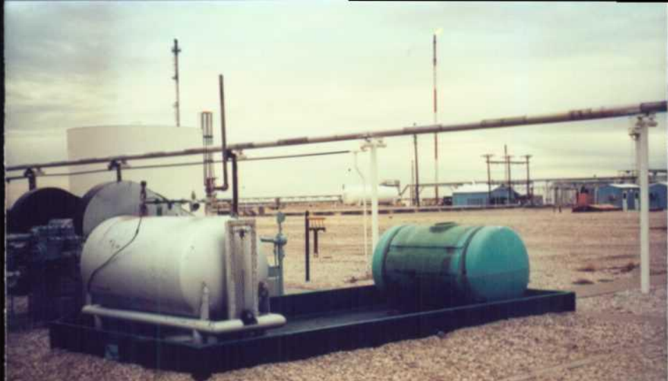
GASSO PUMP USCO OIL & CLEAN OIL. ALCA #4
