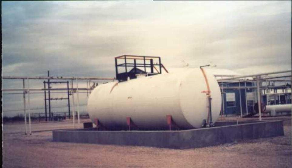
ARCA #6 CLARK ENGINE OIL STORAGE
