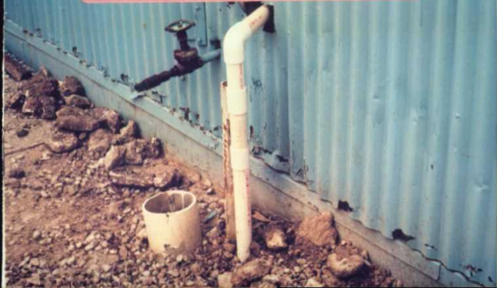
PERMANENT DRAIN IN TREATER
