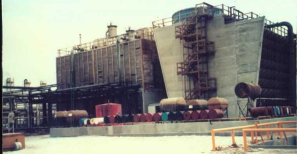
SULFURIC ACID WEST COOLING TOWER
