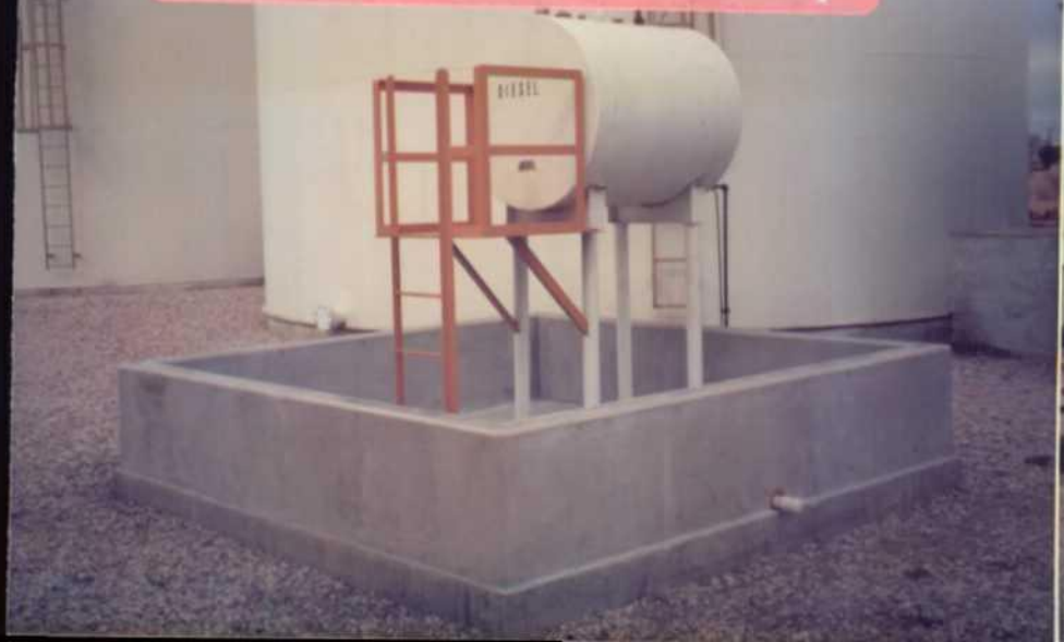
- Fire Pump Fuel AREA #13 -
