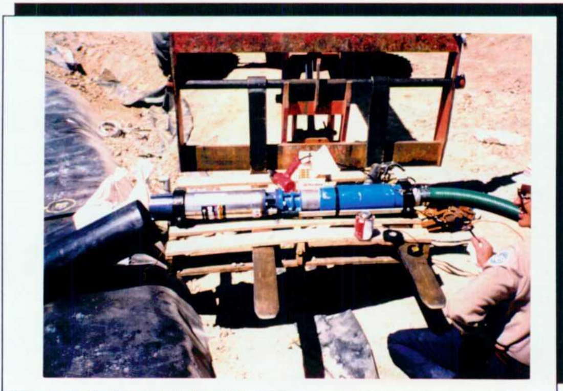
Plate 4 - Well Riser and Submersible Pump
