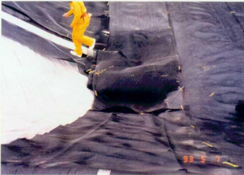
Plate 4 - Leak Detection Sump
