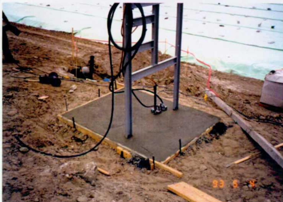
Plate 5 - Control Panel Pad
