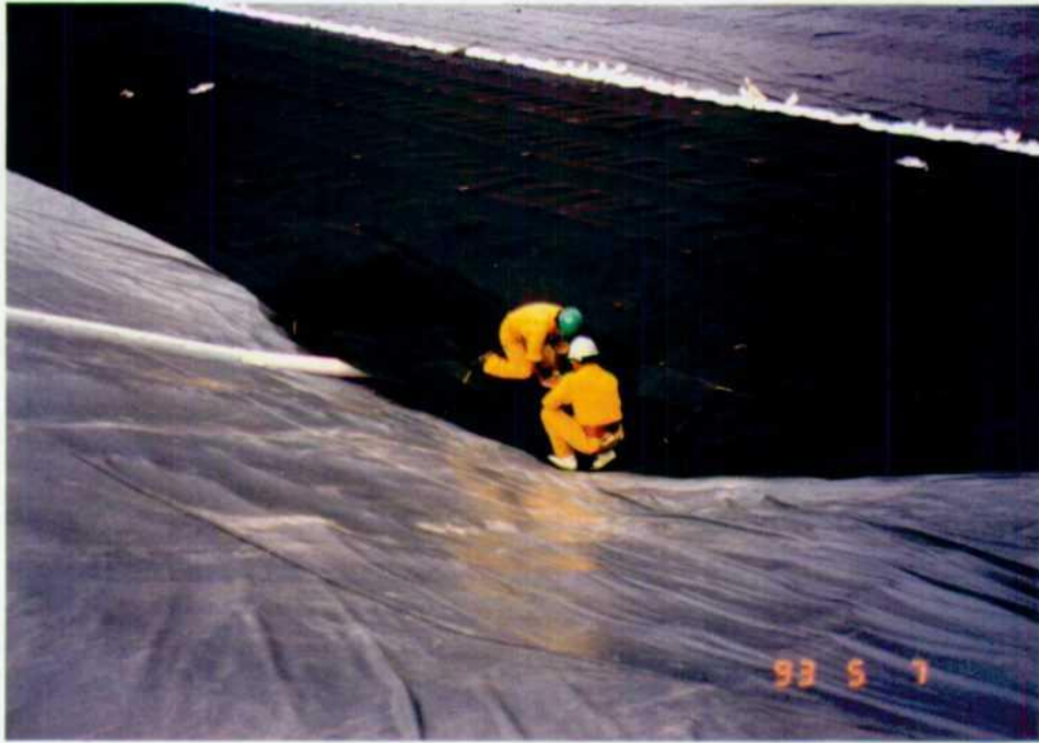
Plate 3 - Leak Detection Sump
