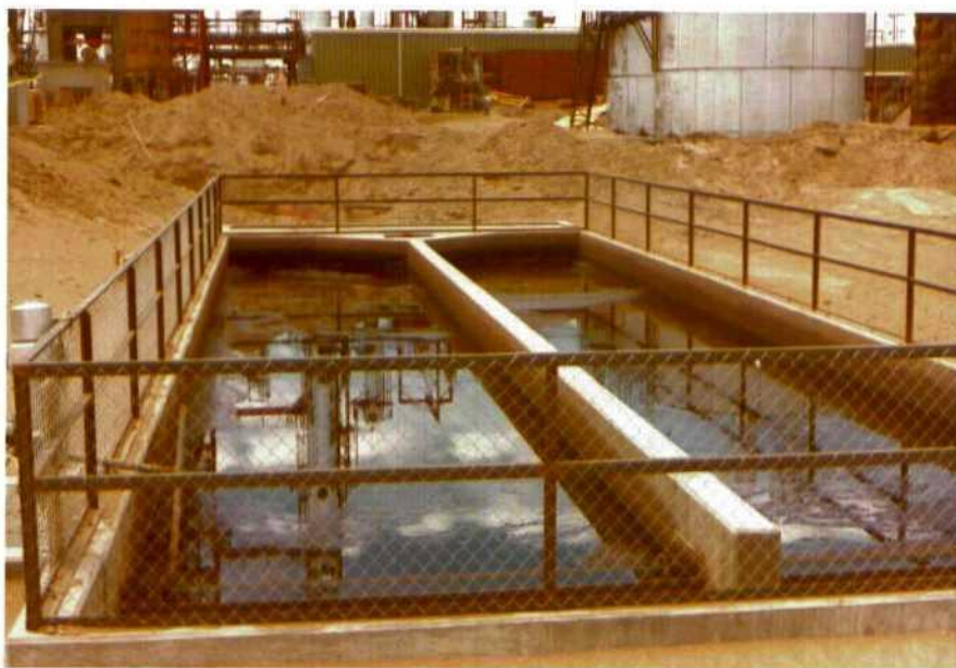
Figure 16. API separator at the Plateau refinery.
