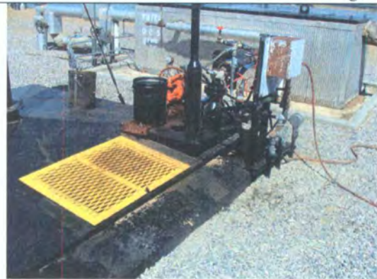
Photo 22: 3 of 3 BGT, leak detection verified dry.
