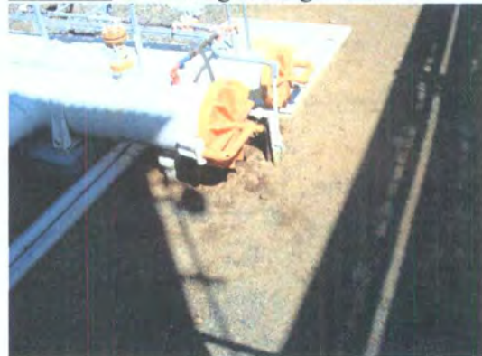
Photo 29: Discharges on ground.
