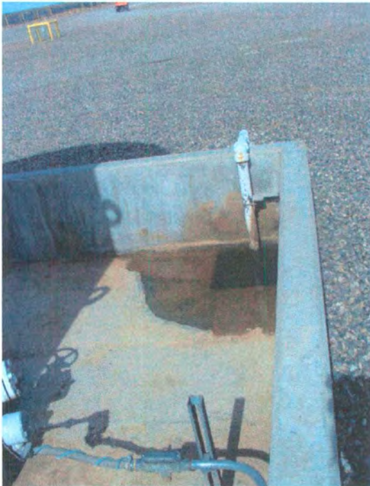
Photo 9: Sump full of fluids.
