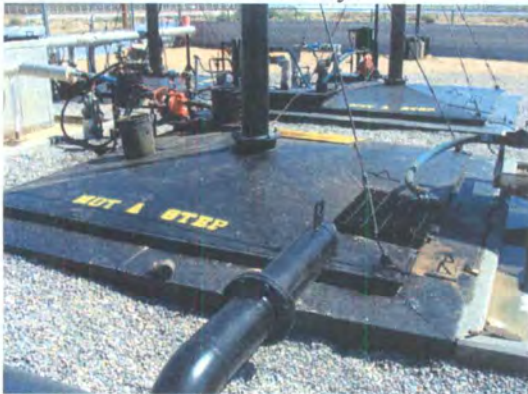
Photo 20: 1 of 3 BGT, leak detection verified dry.
