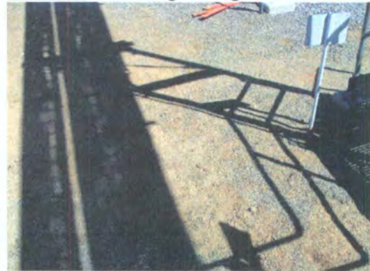
Photo 30: Discharges on ground.
