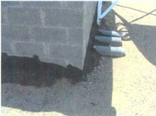
Photo 26: Leaks from secondary containment for filter drain.
