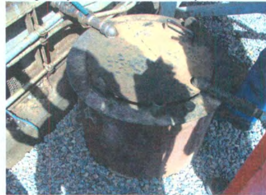
Photo 18: BGT near compressor, leak detection verified dry.
