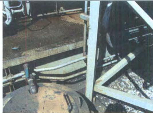
Photo 28: Discharges on ground.
