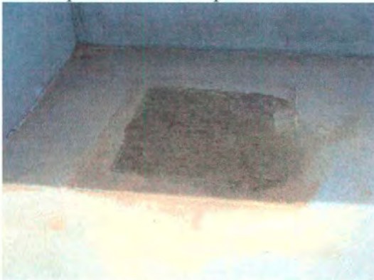
Photo 8: sump in secondary containment full of sediments.
