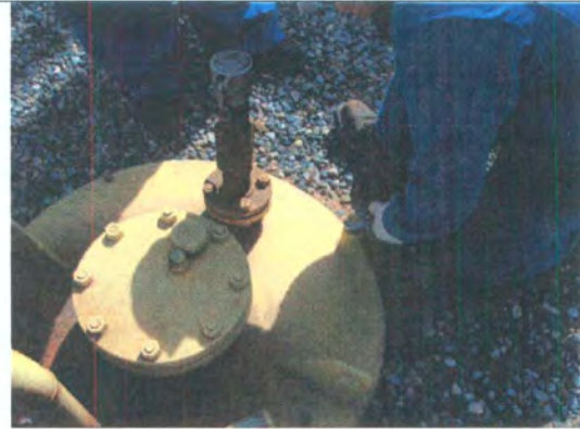
Photo 16: Air compressor BGT leak detection.
