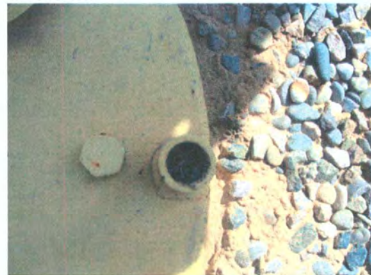
Photo 17: Air compressor BGT, fluids at capacity in leak detection system.
