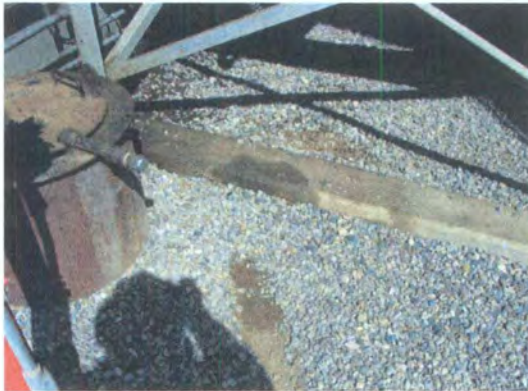
Photo 27: Discharges on ground.
