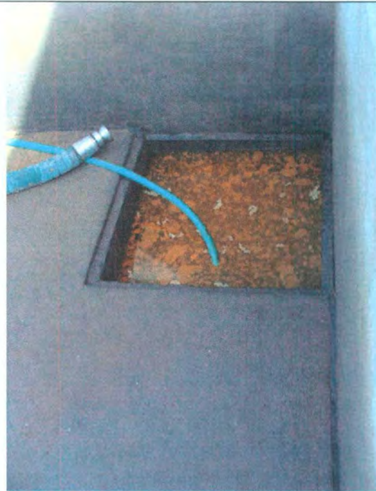
Photo 10: Sump full of fluids.
