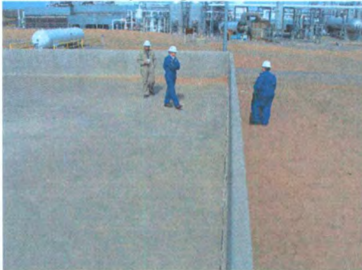
Photo 14: Secondary containment for large Tank 28 & 29 needs work.
