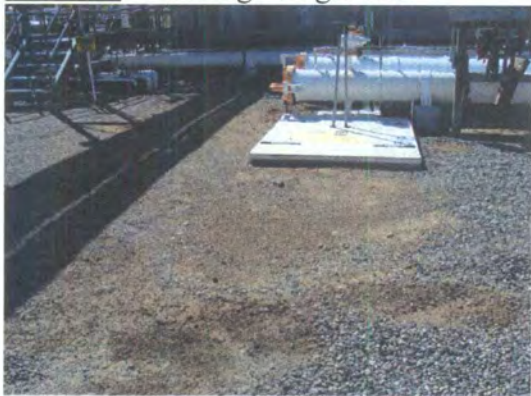
Photo 32: Discharges on ground.
