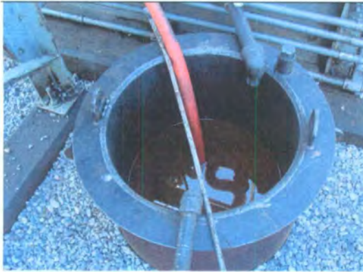
Photo 19: BGT near compressor, no lid. Leak detection verified dry.
