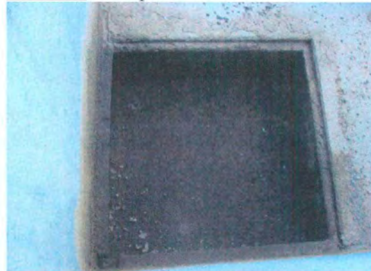
Photo 11: Sump full of sediments.
