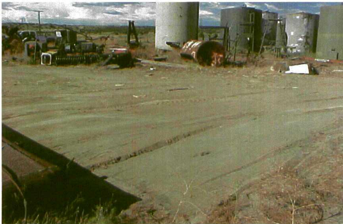
Photo 6: Photograph remaining debris located in cell I-1 and I-2.
