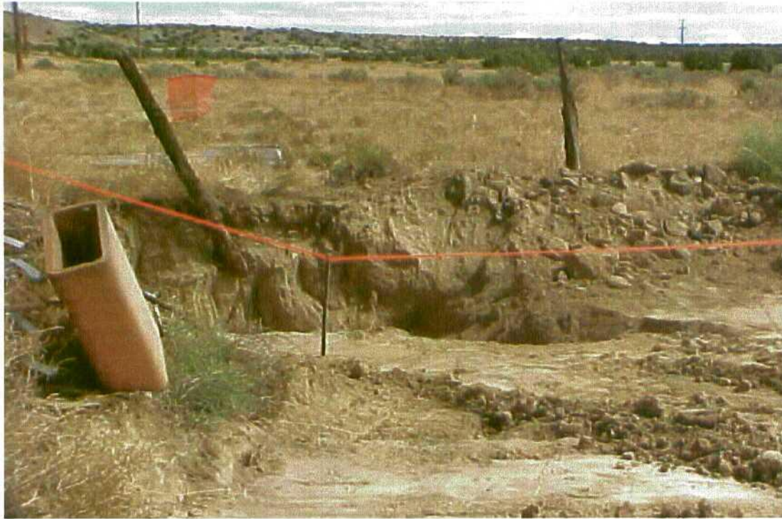
Photo 1: Photograph facing northeast showing an approximate eight (8)- foot deep excavation of a diesel stain.
