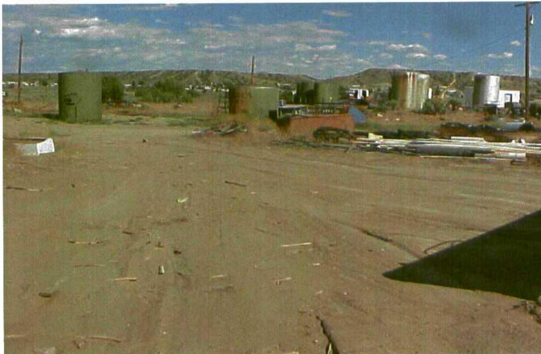
Photo 4: Photograph facing north/northeast showing cells J-3 and J-4 partially cleared of debris and waste products.
