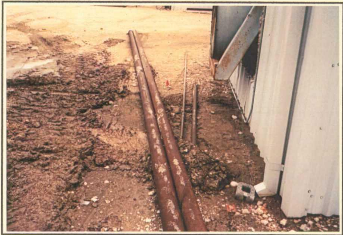
Photograph 12: Sample 1-10 was taken beneath the paint vent located along the north exterior wall of the Machine Shop.
