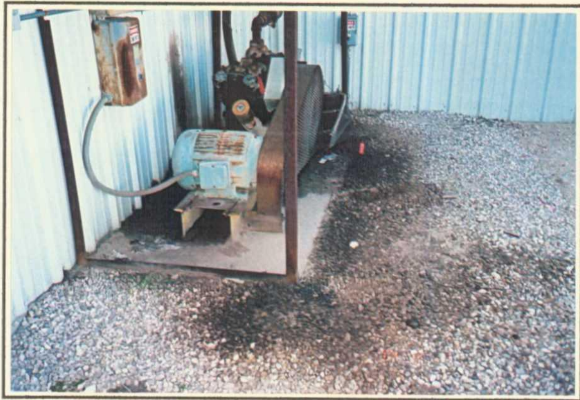
Photograph 4: Soil sample 1-6 was taken at the base of the air compressor concrete located along the north exterior wall of the Machine Shop.
