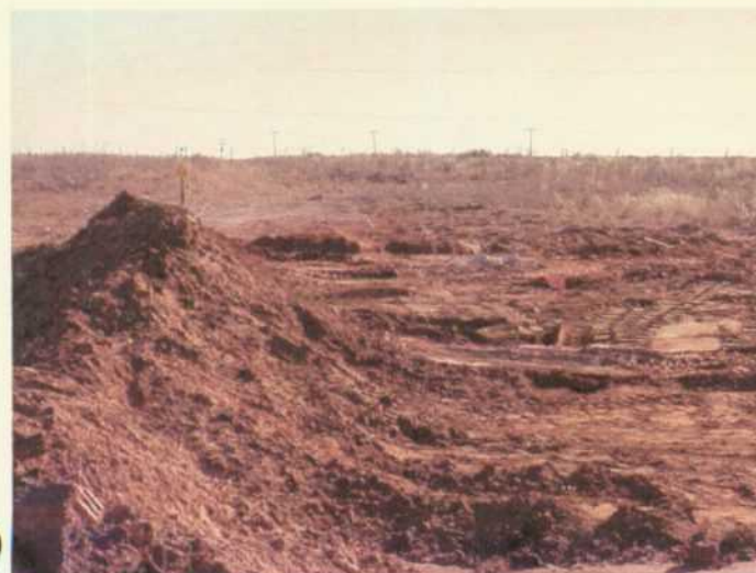
3-11 Looking south at south end of spill
