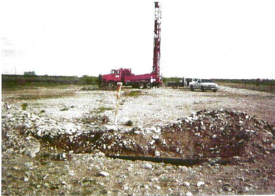
Photo 34: Foreground: Excavated Eott Pipeline located on northern spill site. Background: Drilling of monitor well MW-9.
