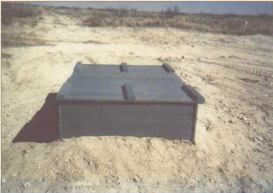
New Junction Box
