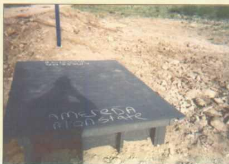
New Junction Box (200' east)
