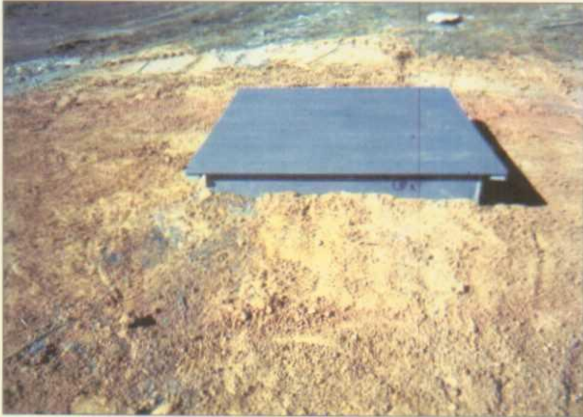
new junction box
