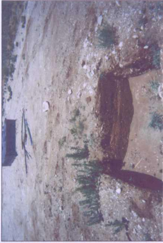
Old Junction Box Site (foreground) & New Watertight Box (background)
