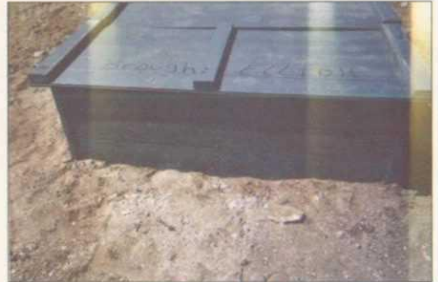
New Watertight Junction Box 45 ft Southeast
