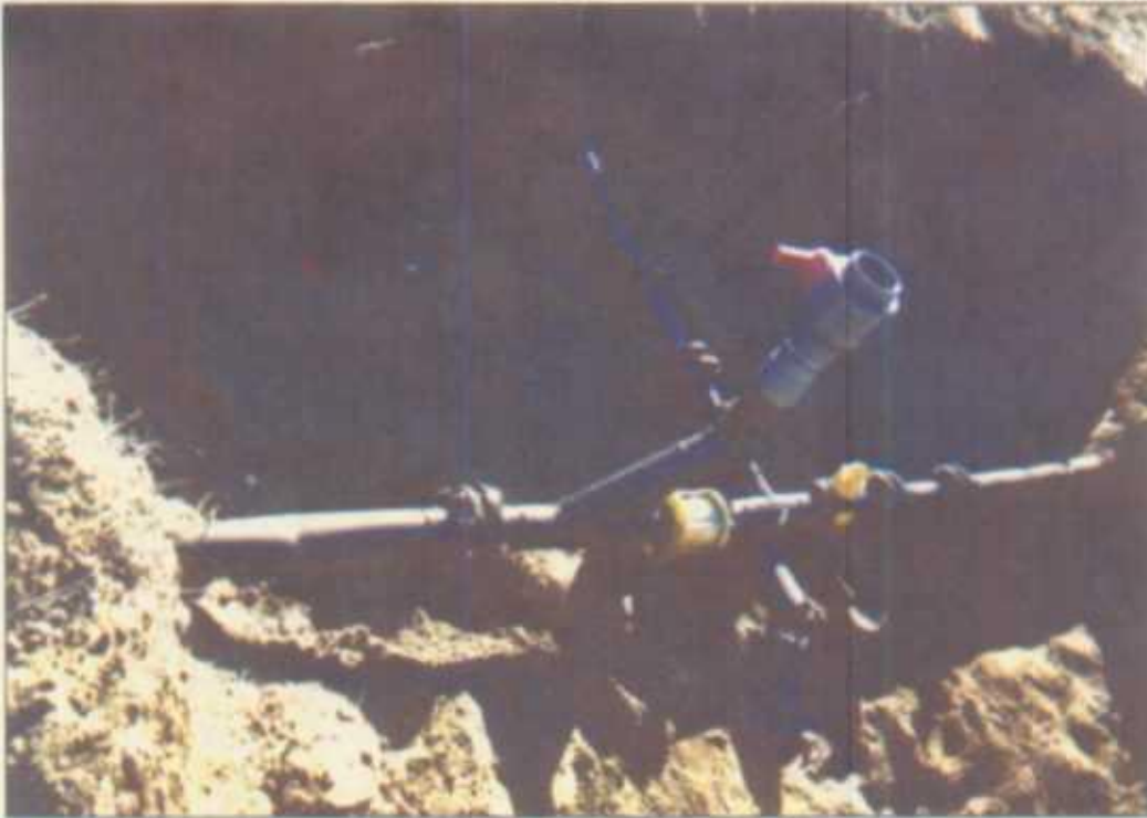
New Plumbing (before remediation)
