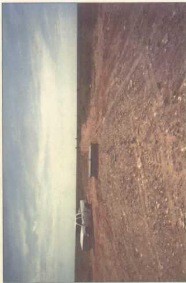
Looking South: New watertight jct. box with ID plate in foreground marking clay barrier below
