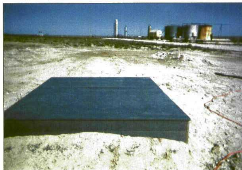
New Junction Box
