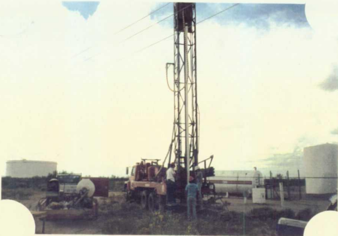
Photograph 1: View of well installation operations on monitor well MW-11 at Lea Station. Note offset tank battery on right in background.
