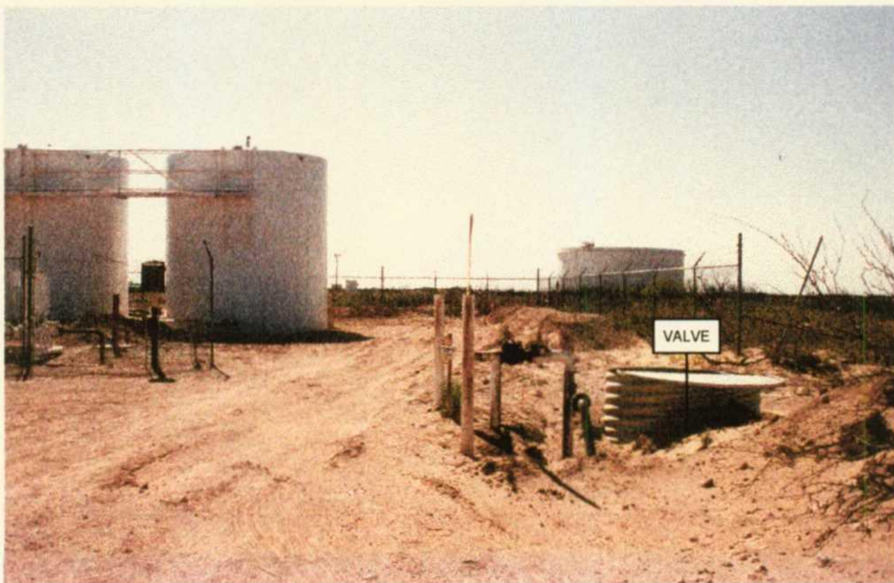
PLATE 2-B - VALVE (SLOW OIL DRIP) TO NORTHEAST OF SUNOCO, INC. (R&M) LEA STATION
