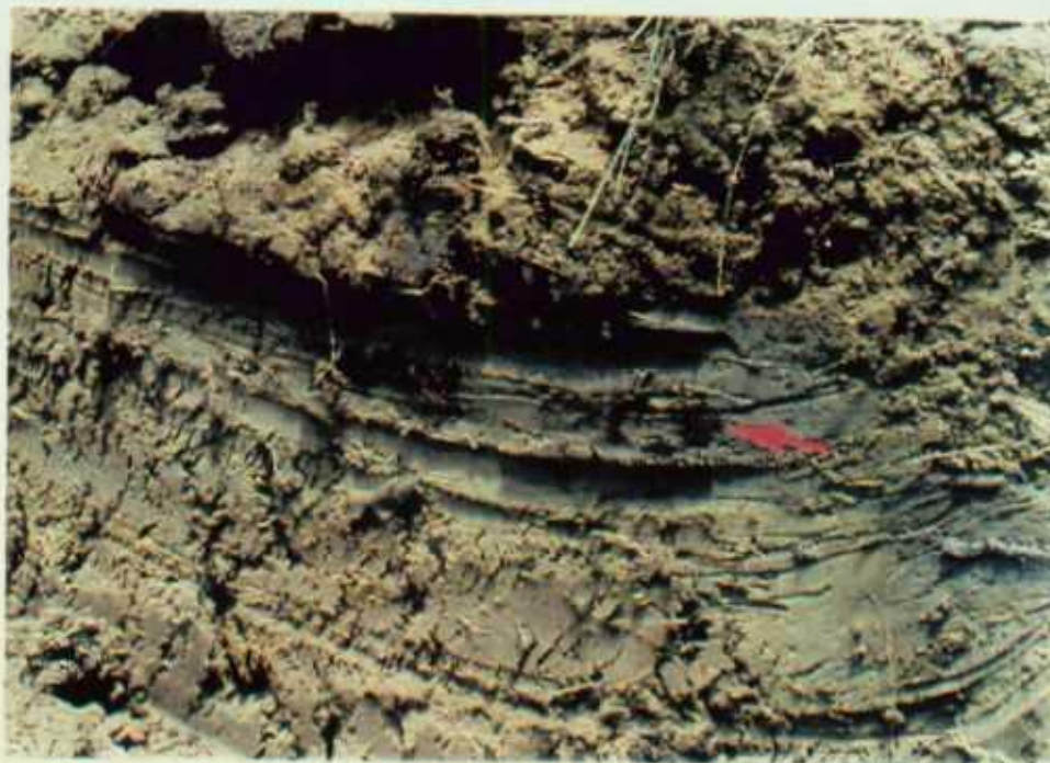
NOTE: CRUDE SEEPING FROM A SOIL VOID IN THE WALL
